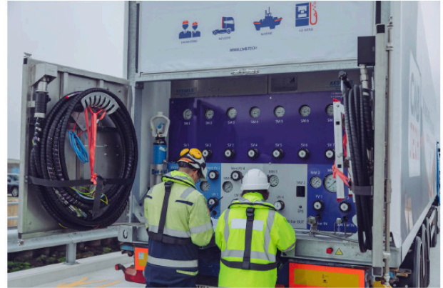
Hydrogen tube trailer bunkering/refuelling panel
