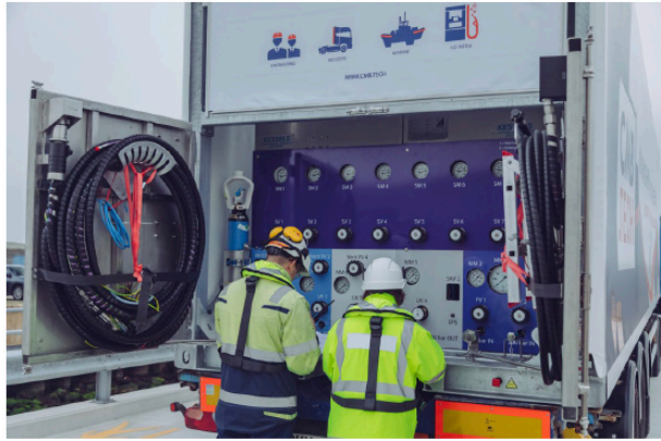
Hydrogen tube trailer bunkering/refuelling panel
